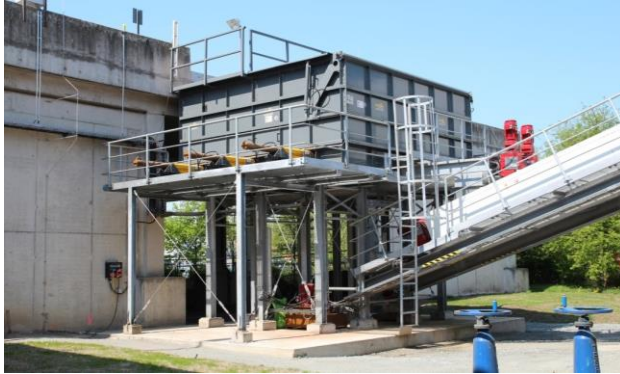
Steel reception container, Bremen power station
