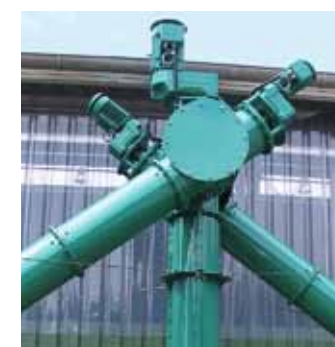
Vertical spiral screw conveyor with 2 alternative fermentation plant feeding screws
