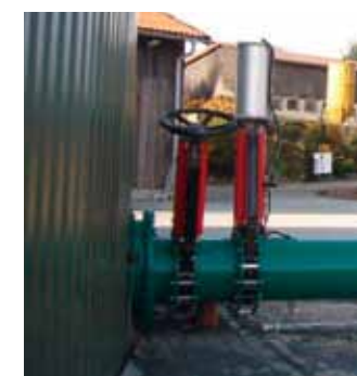
Direct feeding from the solid matter dosing system into the fermentation plant
